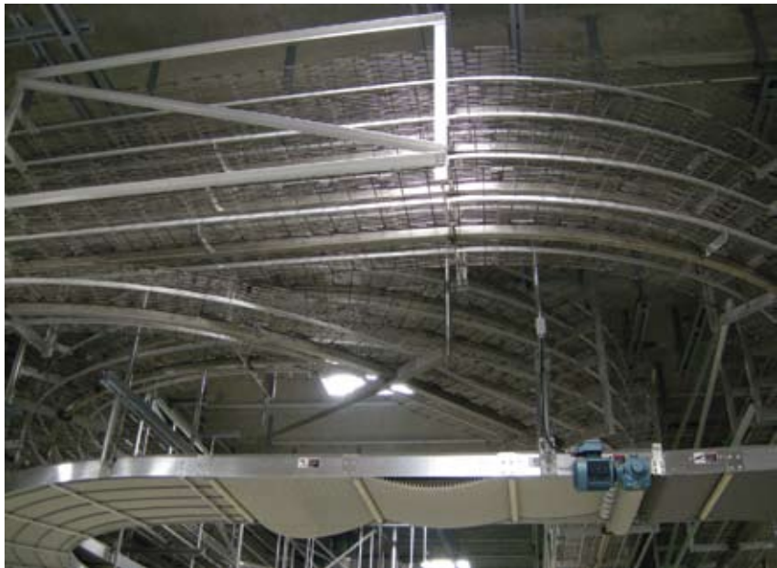
▲ Extra-wide radius turns on the new overhead racetrack cooling conveyors were necessary to accommodate the 40-in.-wide bread and bun pans of the combo line.
